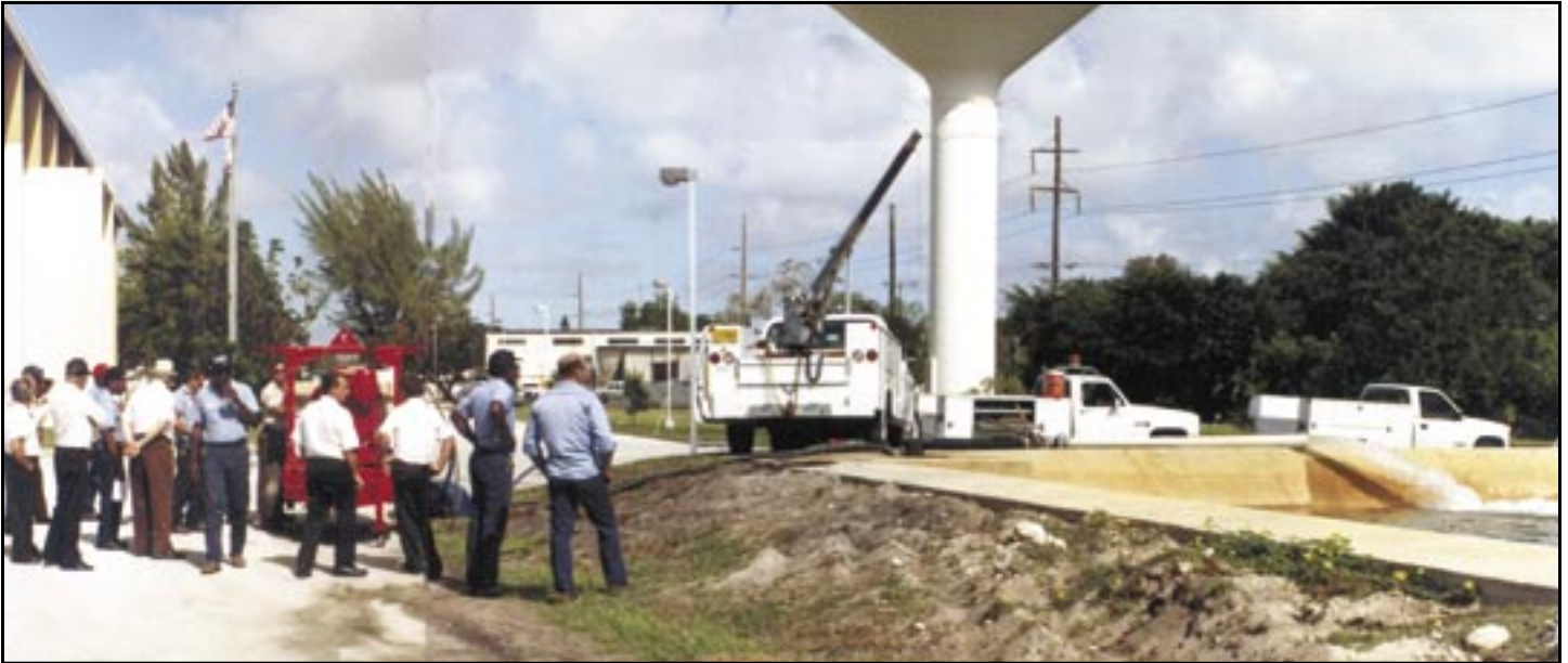
ON SITE TESTING AND DEMONSTRATION OF TRASH HANDLING PUMPING SYSTEM FOR MUNICIPALITY
