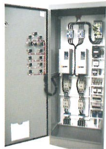
Master Control Center (MCC) soft starting gear
